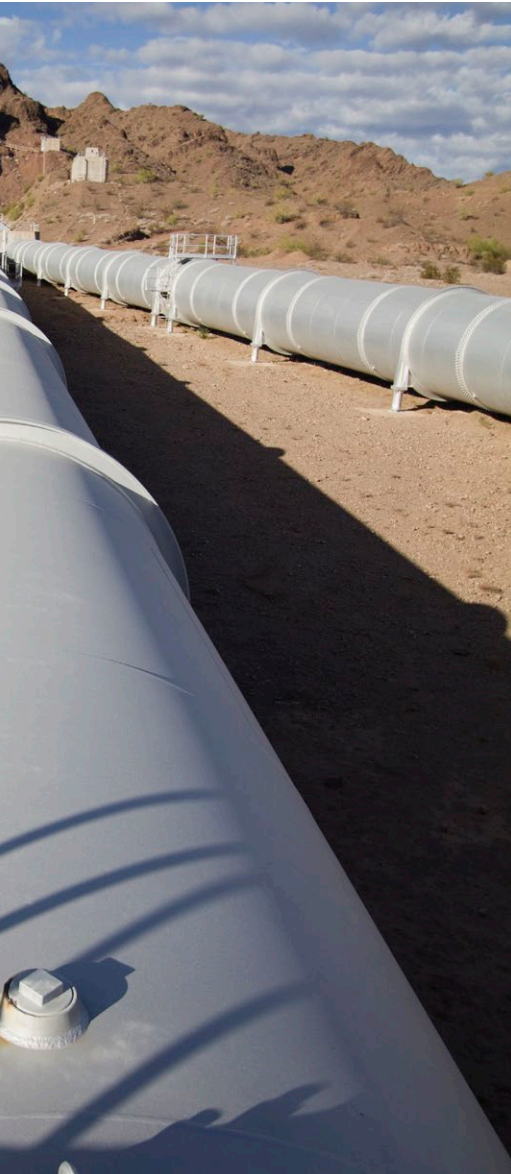
A view from the Gene Pumping Plant.
